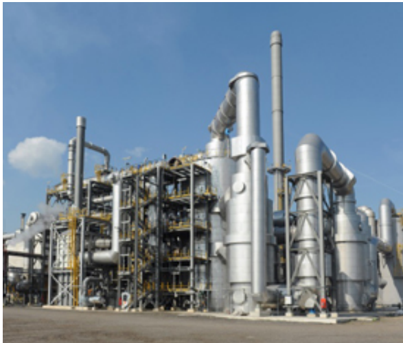
Sulphuric Acid Plant
